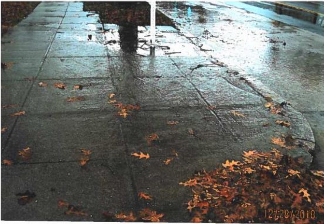
Storm Water Runoff flooding Eastern Avenue sidewalk and curb cut near Metro Bus Stop
