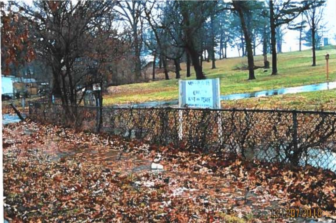
Rear view of property from sidewalk at 3800 block of Eastern Avenue, NE Area flooded with standing storm water runoff
