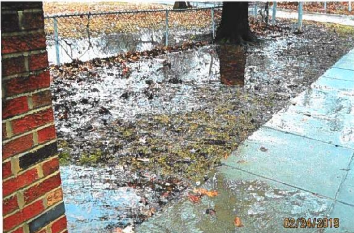
Storm Water Runoff Area next to fence of private property (3814 Eastern Avenue)
