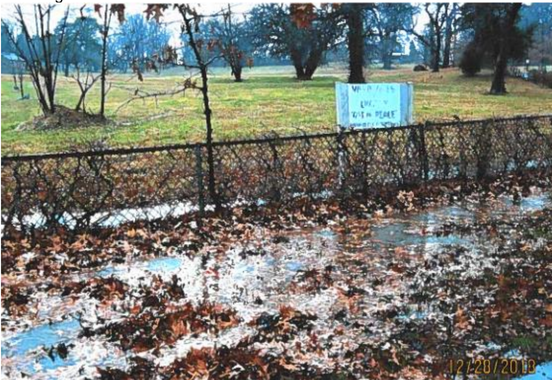
Standing Water at bottom of hill next to sidewalk on Eastern Avenue
